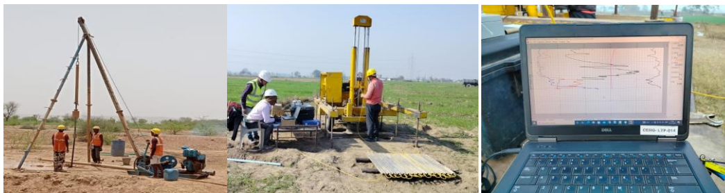
(a) SPT being performed in borehole (b) eCPT in progress (c) eCPT data acquisition
